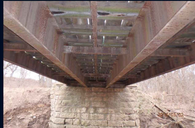
No – not braced.
