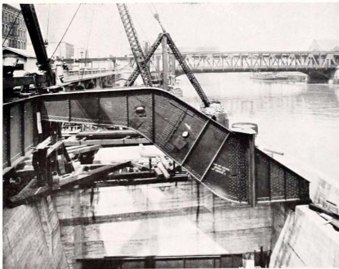
The concrete substructure of the bridge rests on massive concrete piers that are built down to bed rock.
